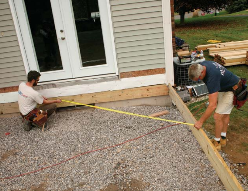
Square up the box. Once the end joists are attached to the ledger, use the Pythagorean theorem to check that they are square to the house.
