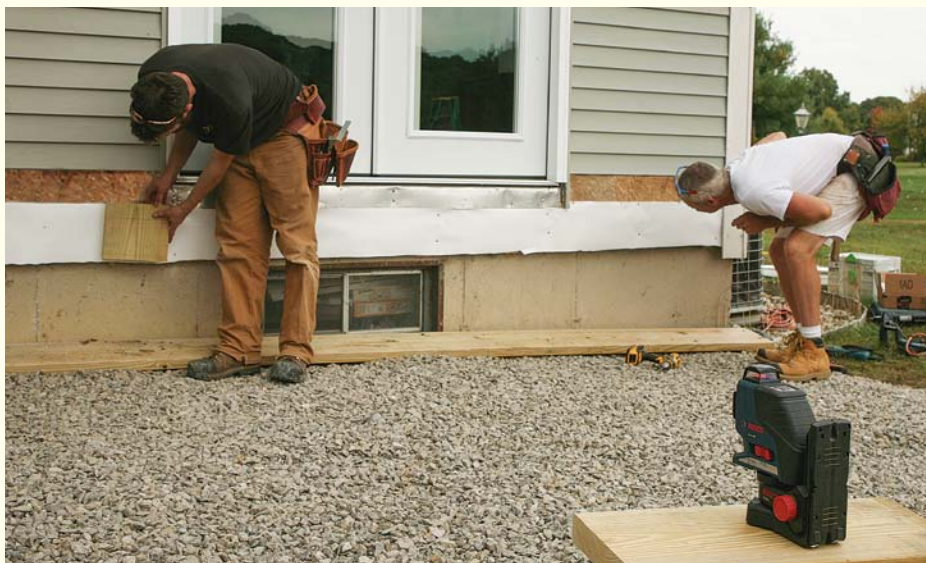
Set the height. After measuring down from the doorsill, use a laser to establish a level line that indicates the top of the upper platform, then snap a chalkline.
