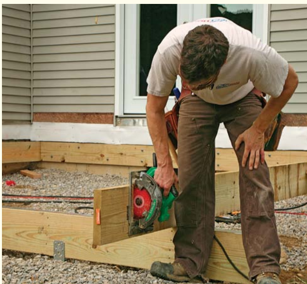
Trim for the rim. Taking the foundation's jog into account, cut the end and center joists to length.
