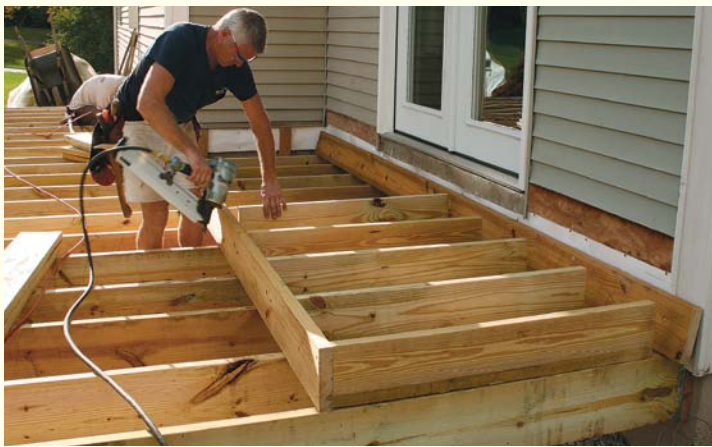
Framing the platform on the deck ensures accuracy. Align the platform joists with those on the deck during assembly.
