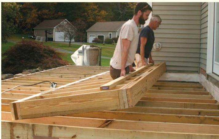
Not a drag. After applying a liberal bead of construction adhesive on the deck-joist tops to prevent future squeaks, slide the platform into position, and toenail it to the frame below.
