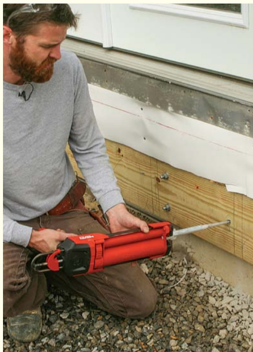
Glued to the foundation. Attach code-mandated lateral-load hardware (Simpson DTT2Z or similar) with construction-grade epoxy and 1/2-in. galvanized threaded rod.
