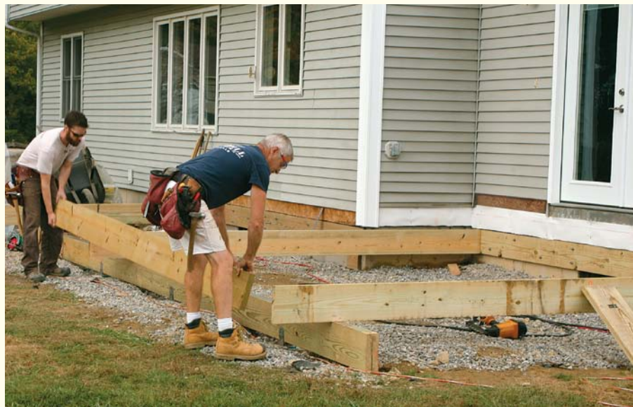
Attach the rim. Nail each half of the rim joist into the joist ends with 16d galvanized common nails. Because the ledger was straight, the joists were gang-cut to length.
