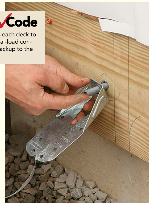
Hanging around. Once the epoxy has set, it's a good idea to loosely attach the lateral-load hardware to the rod so that it's not forgotten.
