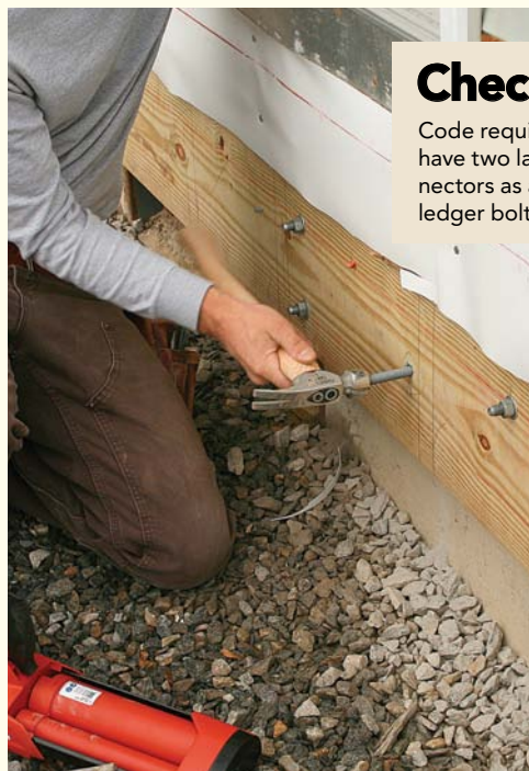
Push, don't strike. The threaded rod used to attach the hardware needs to be held firmly in place for 30 to 60 seconds until the epoxy firms up.
