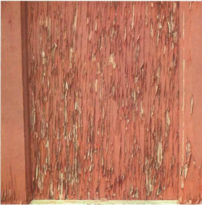
Moisture absorbed into the surface checks of the plywood caused this paint to peel. Exterior plywood should be painted with an acrylic-based paint, which is flexible and resists cracking caused by the seasonal movement of the plywood veneer.
