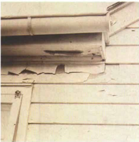
Excess moisture causes peeling paint. Leaking gutters and roofs, ice dams and inadequate overhangs are some of the typical causes of peeling paint.
