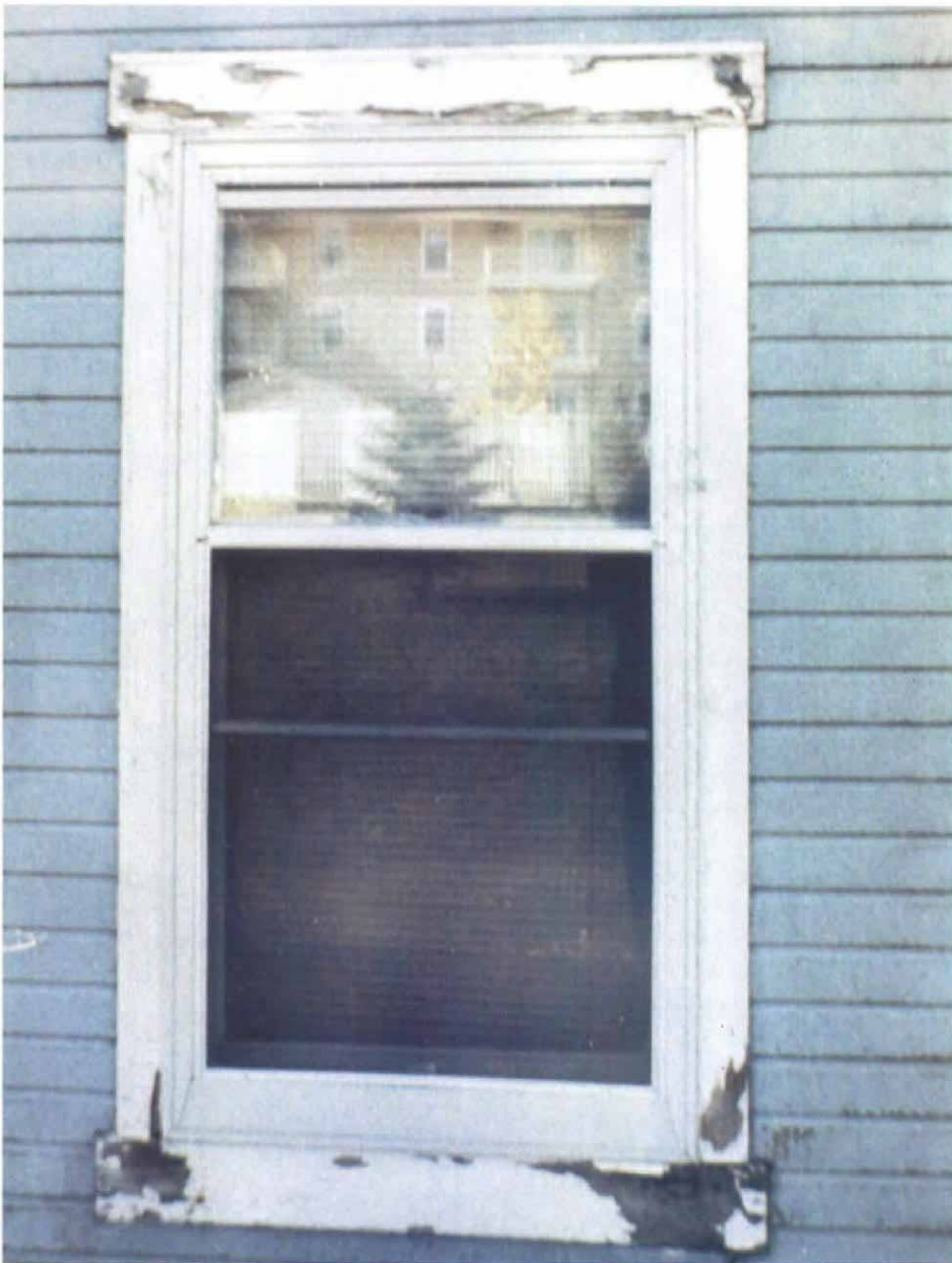
Moisture from the inside will cause peeling paint on the outside. Moisture-laden air escaping from around a leaky window will cause paint to fail at the point of exit.
