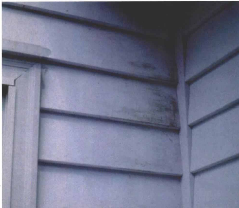
Discoloration can be an early sign of paint degradation. This protected corner shows the early stages of paint degradation caused by interior moisture. Typically, the stained areas will begin to peel if the moisture's source is not eliminated.
