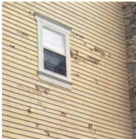
In need of a vapor barrier. In many older homes, the combination of moist air leaking out through walls and inflexible layers of paint causes peeling and cracking.
