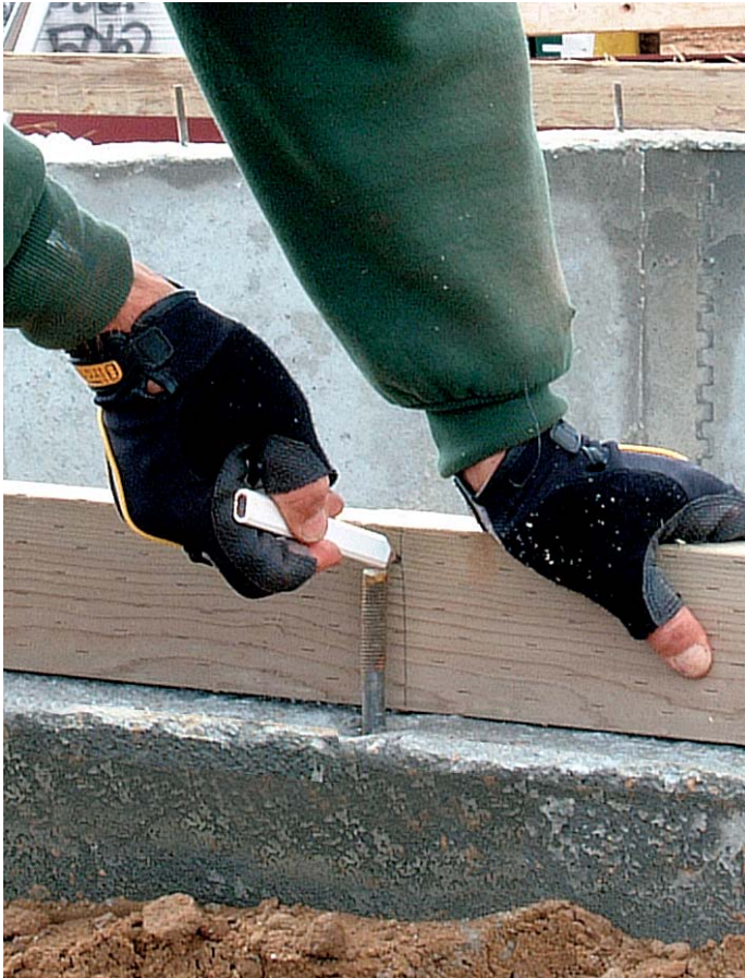
Stand the sill plate on edge and trace the outline of the bolt onto the plate.
