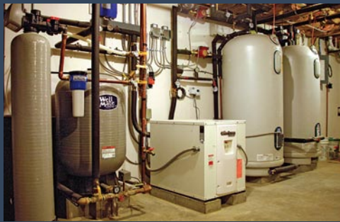
The heart of the system. A heat pump extracts heat from well water. The extracted heat is stored in two 100-gal. electric hot-water tanks—one for the radiant-heat system and one for domestic hot water.
