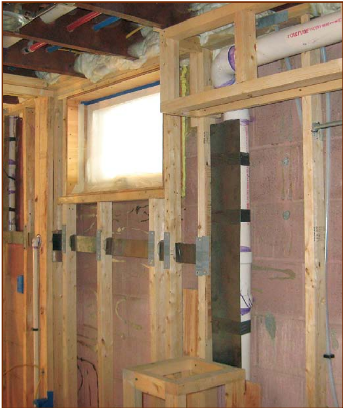
A better basement wall. The basement of the 1960s ranch was typical of the era—damp, cold, and uncomfortable. To insulate the original block foundation, we framed new 2x3 stud walls 2 in. away from the original block wall. Filling the resulting 4½-in.-deep cavity with closed-cell spray foam yielded an improved foundation assembly of R-27.
