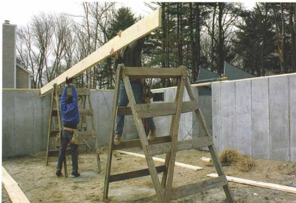
Up, over and into the pocket. Preassembled beam sections are easy for two crew members to lift. Here, crew members slide one end of the beam into the foundation pocket and rest the other end on the A-frame scaffolding.
