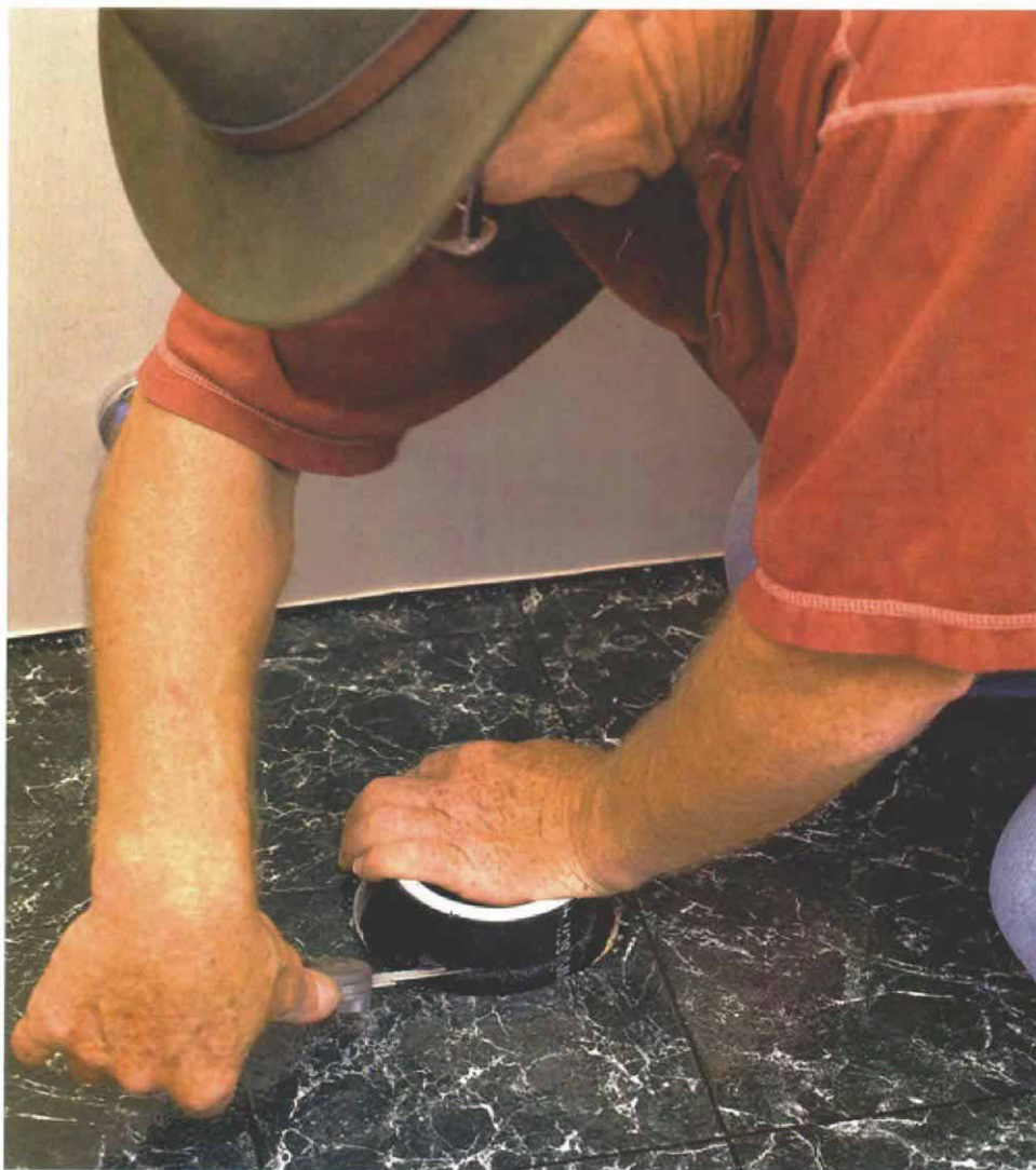
Trim the drain line. The author uses a small handsaw with a reciprocating-saw blade to cut the plastic drain pipe flush with the floor. The white ring atop the pipe is the remains of the test plug.
